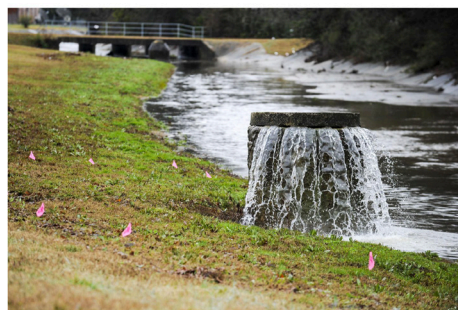
Untreated sewage pours from a manhole on Central Parkway Southwest on Dec. 23. The same manhole contributed to the 1,680,021 gallons in sewage that escaped the Decatur Utilities system over the last week. (JERONIMO NISA/DECATUR DAILY FILE)
